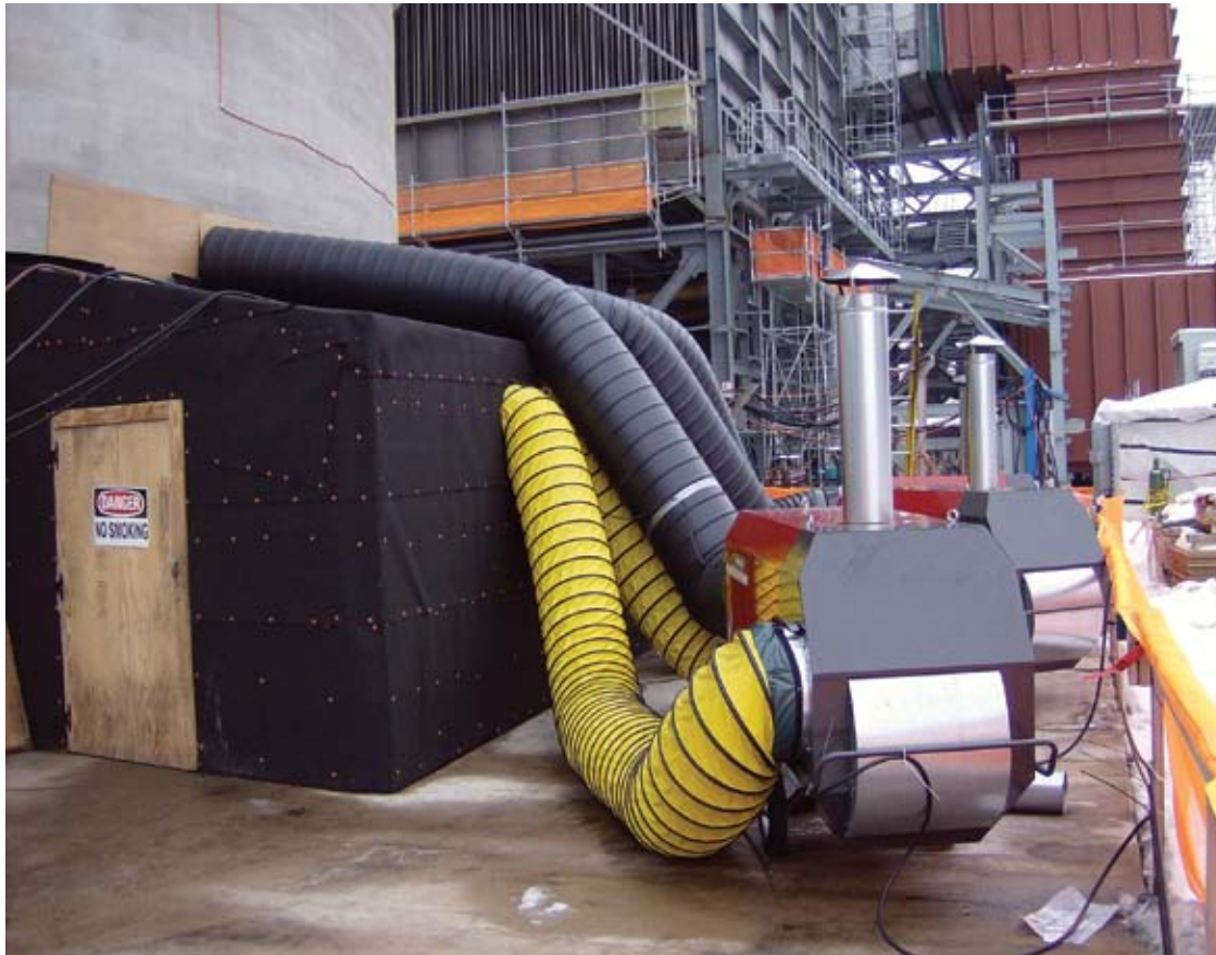
« A 700,000-Btuh, indirect-fired portable heater is shown here being used to heat a construction site. Return air is recirculated through the heater to form a closed loop.
