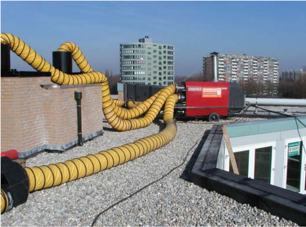
« Fresh outdoor air is heated and then ducted to multiple areas to warm this construction site.
